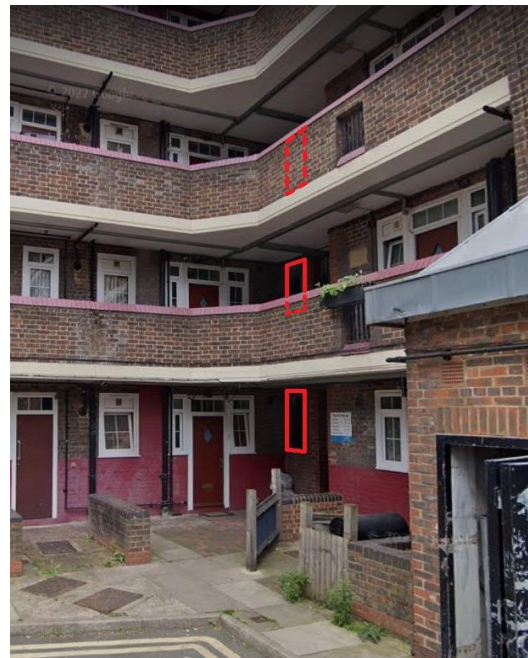
Image 41 (above): Photo of Rennie House, overlaid with the outlines of three of the five bedroom windows that would experience substantial adverse VSC percentage losses.
